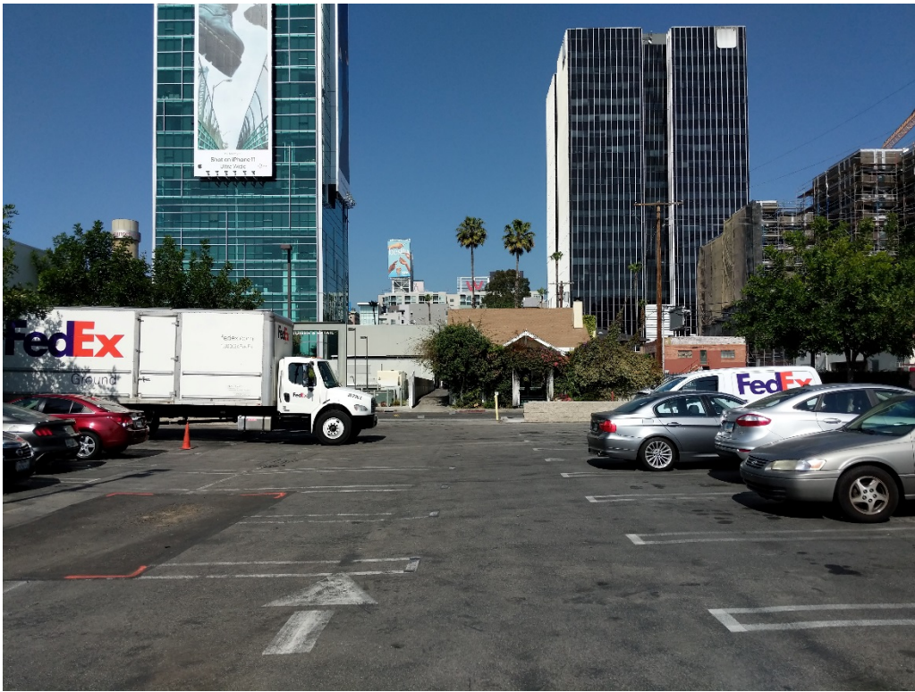
View of parking area showing an area of patched asphalt. 1400 & 1440 Vine Street, Hollywood, California 90028
